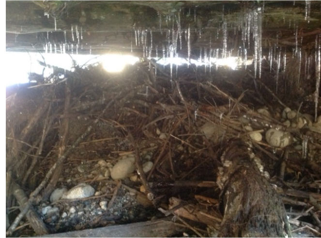
debris under structure
